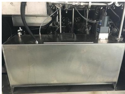
Pipe and valve
